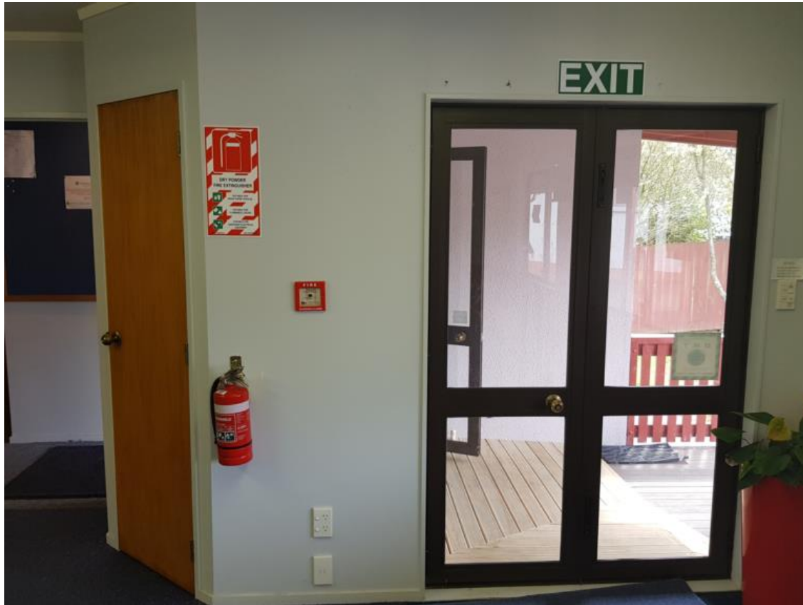
Fire Exit/Call Point & Fire Extinguisher at the Parish Hall Kitchen
