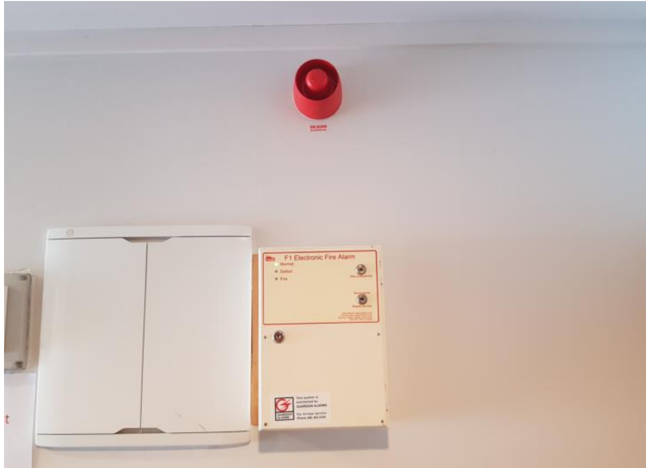
Fire Alarm Panel at the Parish Hall Kitchen
