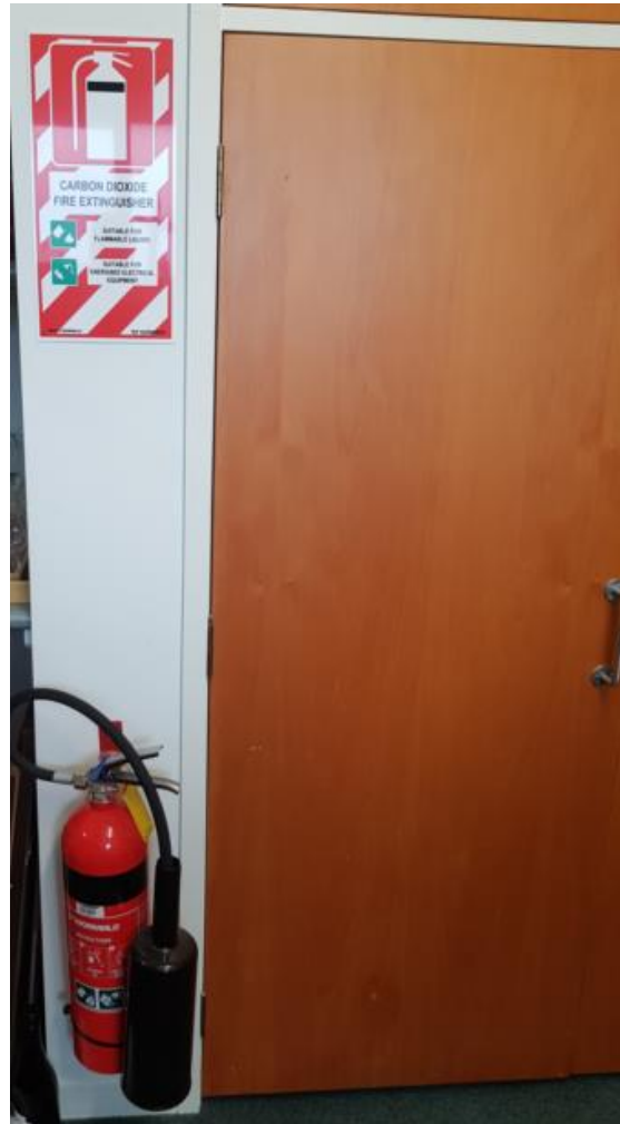
First Extinguisher inside the Sacristy
